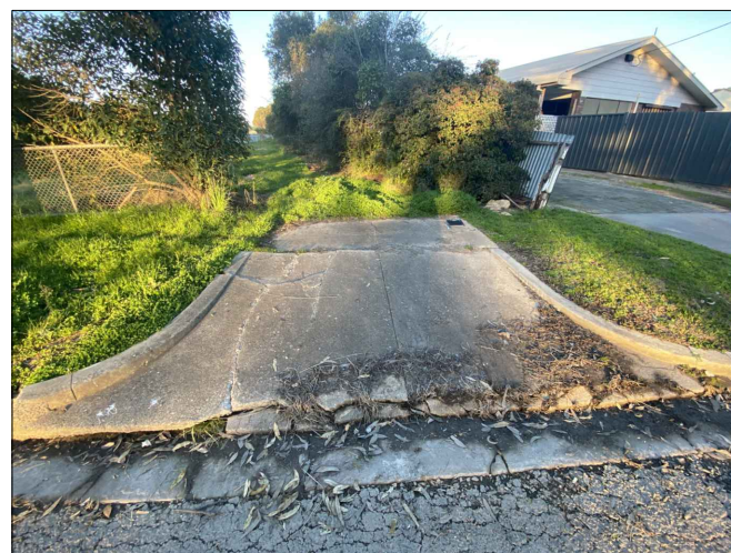
Damaged crossover to subject site.
