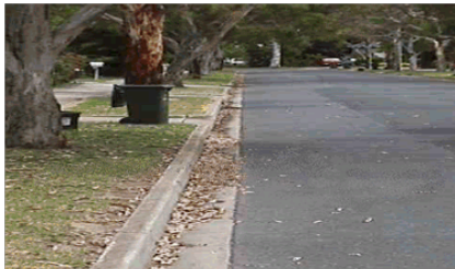
Condition 3 - Old but only Minor loss of shape & movement
