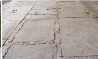
Condition 7 - Extensive cracking and movement
