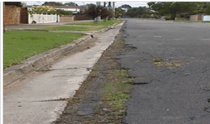
Condition 6 - Movement and Concrete breakdown
