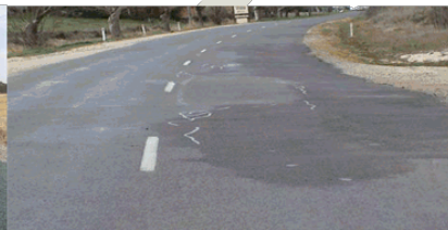
Condition 6 Moderate failures and shape loss
